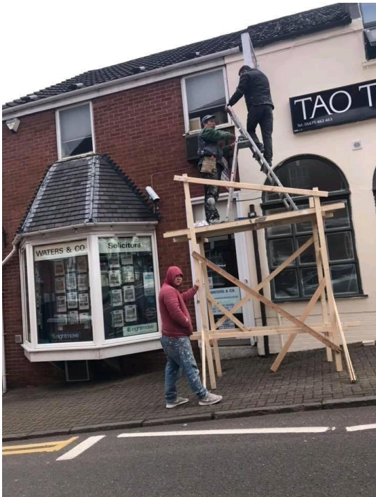
No Scaffold Access
