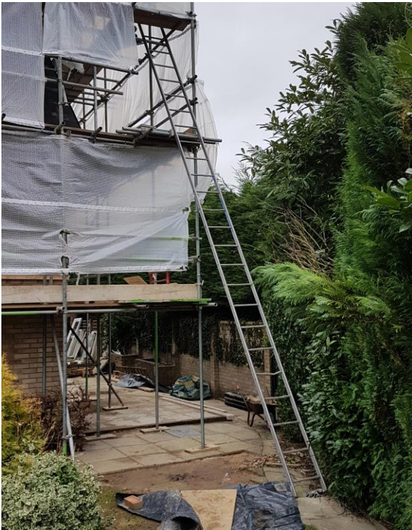
Spot the hazards!
